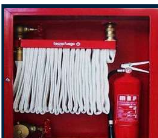
Gabinetes y Mangueras Cabinets and Hoses
